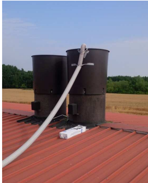
Figure 1: Exhaust duct of the ventilation with flexible tube for sample gas
