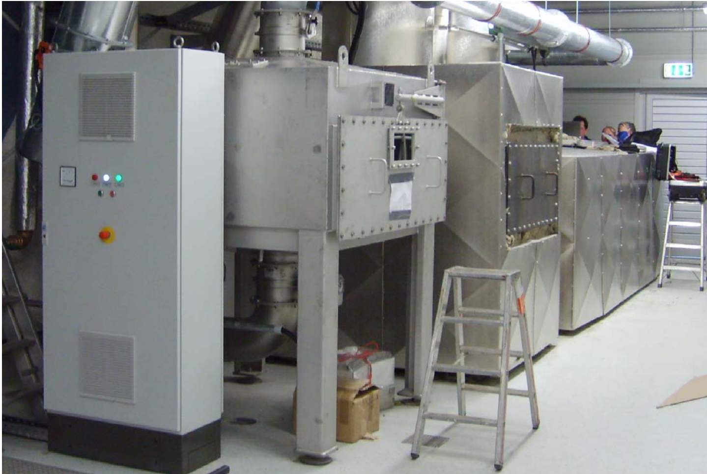
Figure 11: Catalytic supported NTP plant for 10,000 m 3 /h of waste air behind flavouring processes for food
